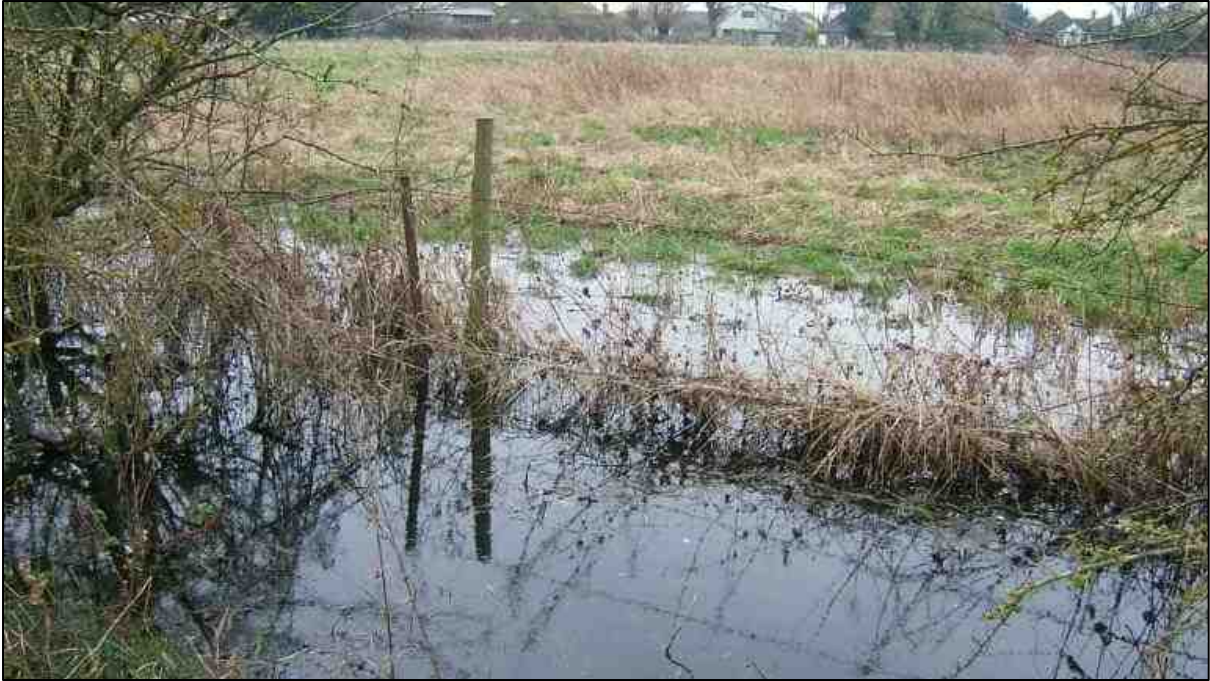
Figure 7: The ditch flowing along the western boundary of the Pye Homes site, currently exceeding capacity with the houses on Milton Road in the background.
